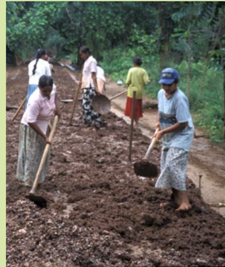
Women spreading a fine gravel as the surface layer of a community road, which will be rolled in later.
